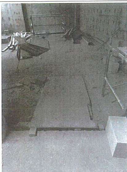
斜坡通道木板未钉牢固
